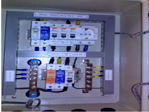
Gambar 3. Panel lightning Arrester
