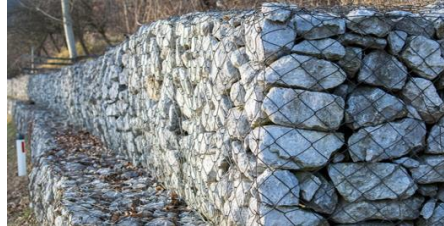
Gambar 6. Dinding Penahan Bronjong (Gabion)
